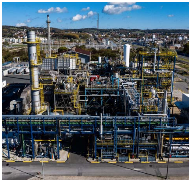
Air Liquide's innovative technology, Cryocap, demonstrated at industrial scale in Port Jerome, France, enables the capture of CO 2 from a hydrogen production unit via a combination of cryogenic and membrane processes. (Copyright: Adrien Daste)
