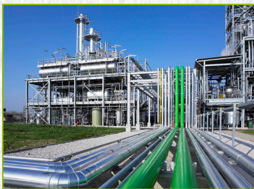
Biofuels Production Unit – Spain
