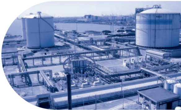
Fos Tonkin - Integration of Air Liquide Air Separation Unit with the LNG terminal (exchanger LNG/N 2 highlighted)
