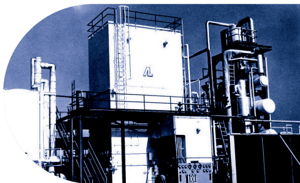
Air Liquide designed Memphis Peak Shaver 5 MMscfd
