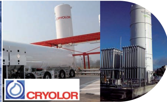
Cryolor, a subsidiary of Air Liquide provides LNG satellite station and the biggest 78,000L jumbo LNG trailers
