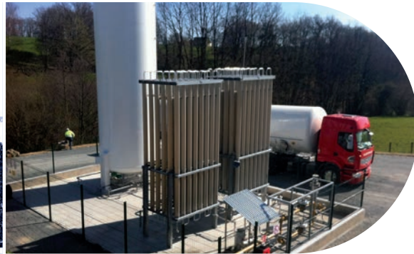
Air Liquide atmospheric vaporizers on Valade Lubersac satellite station
